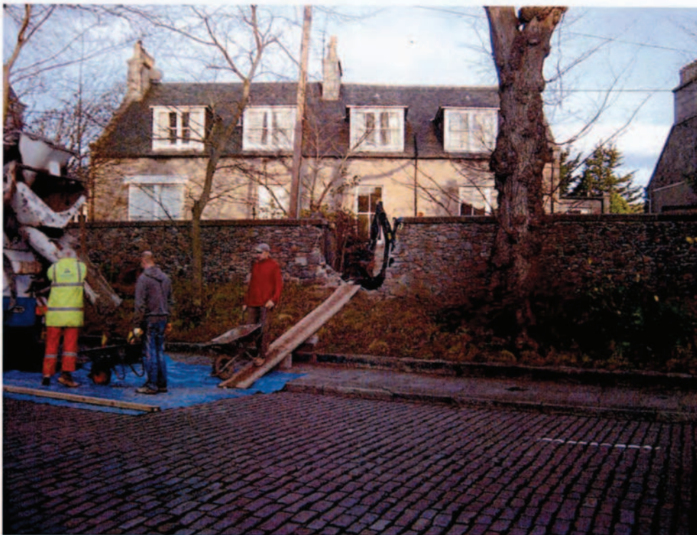
Photo 6 Another Breached wall in Albert Terrace / Carden Place – this time to allow 'change of use' from Residential to Office Accom.
